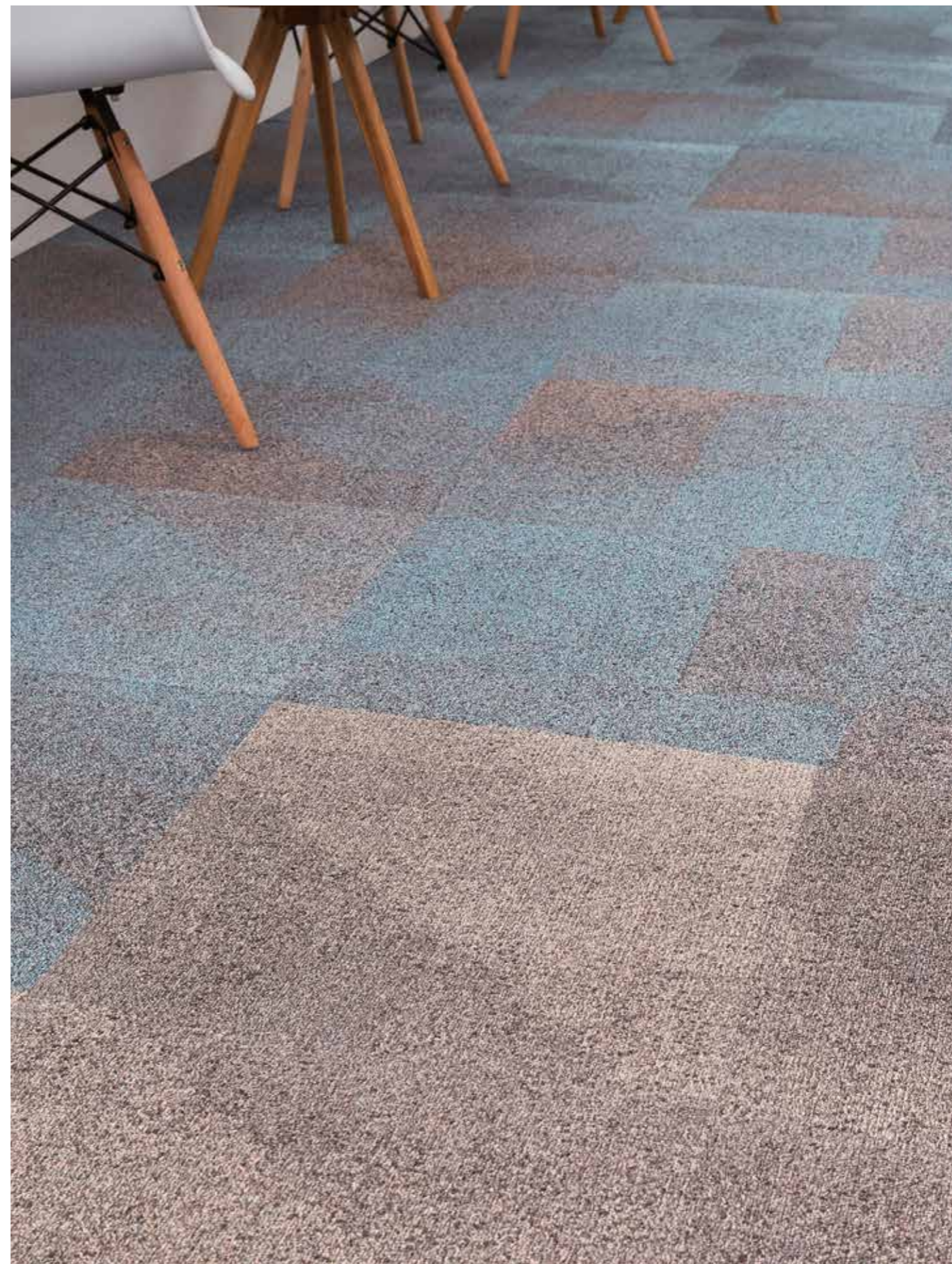
Beyond in Arctic B, Mulberry Arctic B and Mulberry B, custom installation
