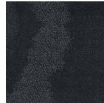
WAS154-133 TAR (Burned BUR154-133, Distressed DIS154-133)
